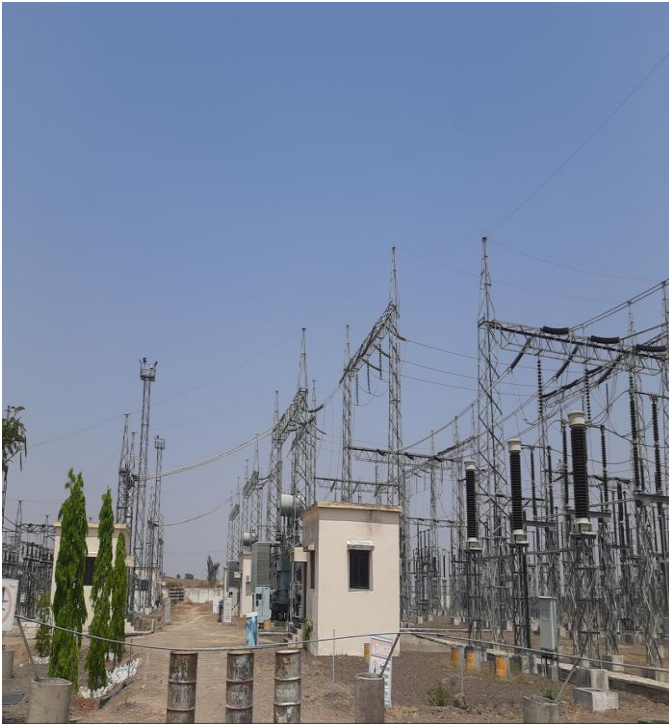
220/33 kv Khanapur PSS
